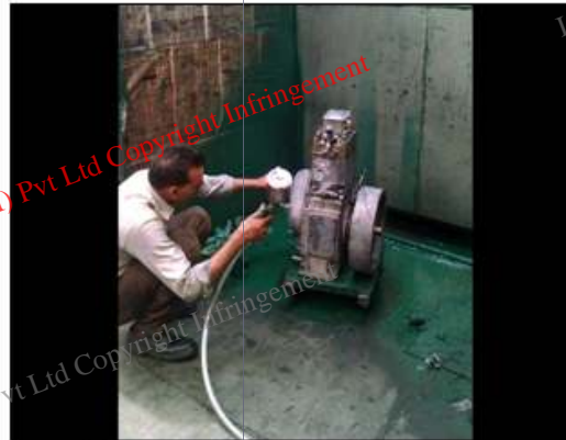
Wrong Paint Booth Design
